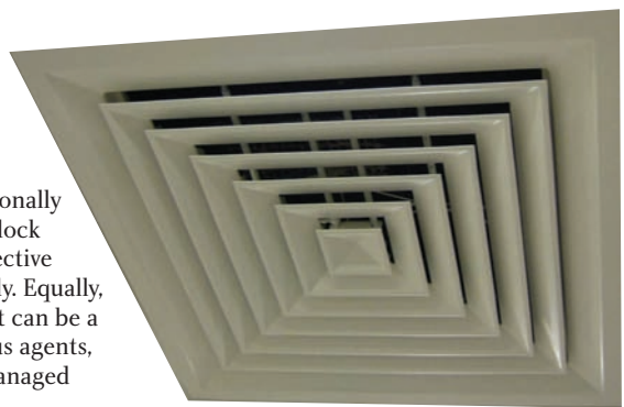
MRSA can easily circulate through the air supply and return via ventilation systems.
