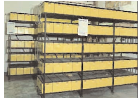
Figure 3: Stand mounted batteries for a UPS system protecting a central IT room.
