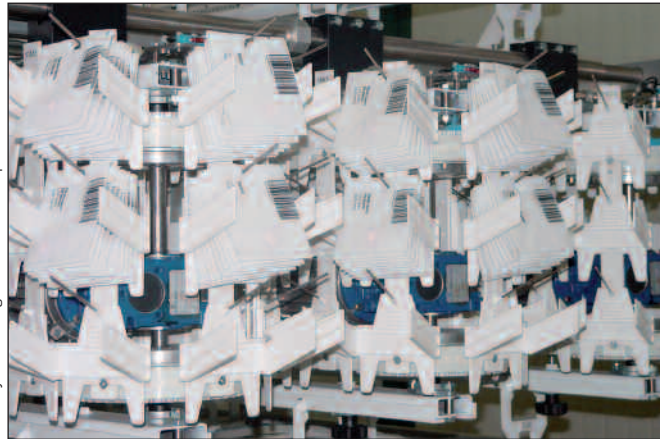
The hospital is benefiting from two PillPick automated drug management systems, installed within the existing pharmacy.
